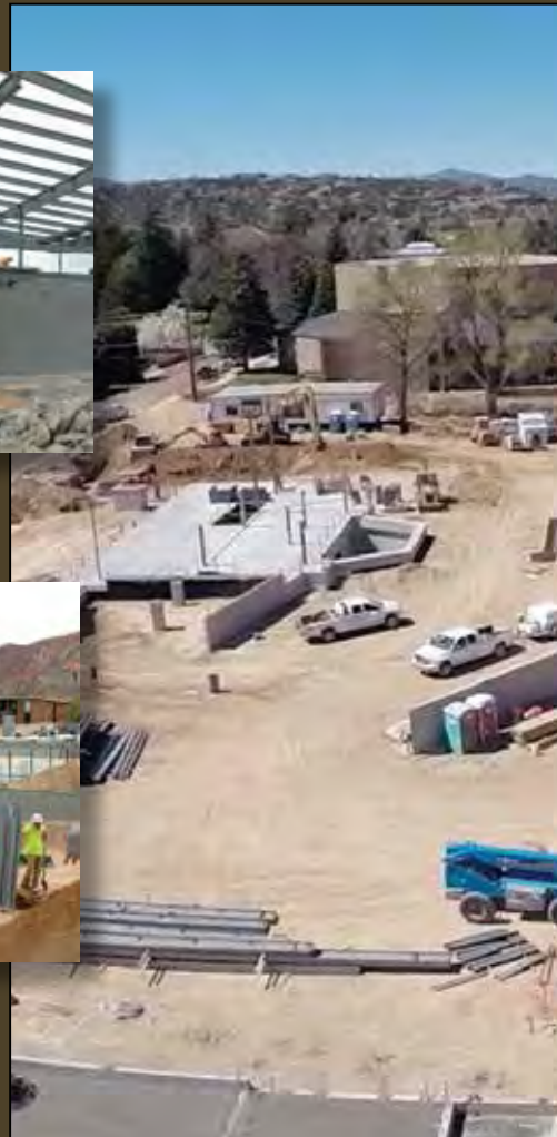
Aerial view of the construction of the Beverley Taylor Sorenson Center for the Arts.
