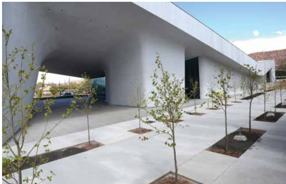
The Southern Utah Museum of Art in the final stages of construction (April 29, 2016).
